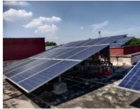
Solar PV installed on building roof
